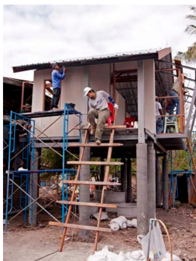
A new home built on stilts to mitigate against future flooding in Lopburi.
