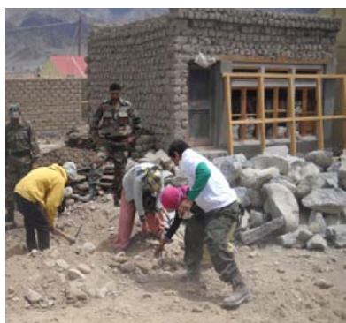
Homeowners and soldiers-volunteers lay out the foundation for a new home, then dig it.
