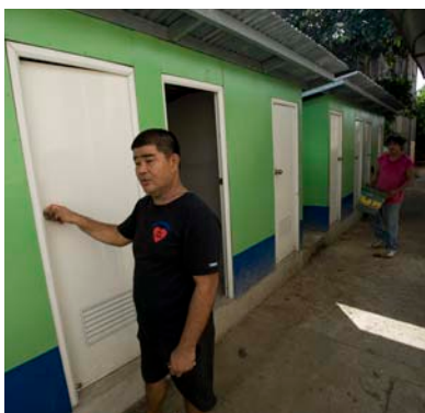
Workers finish 20 toilets at Malanday Elementary School. New kitchen units were also part of the pilot program.
