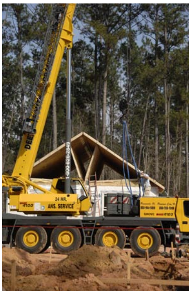
Modular houses are built in a factory and transported to a lot. A crane places the modular on its permanent foundation.
