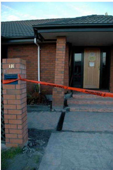
A damaged house after the earthquake.
