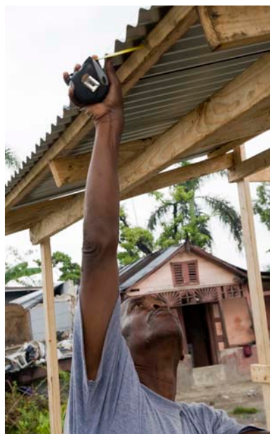
A worker helps to build the first 10 Habitat for Humanity transitional shelters in Léogâne, in the Kada neighborhood.
