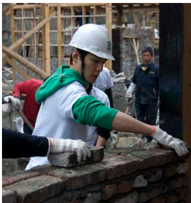
Top: Earthquake survivor in front of a two-story housing solution under construction.
