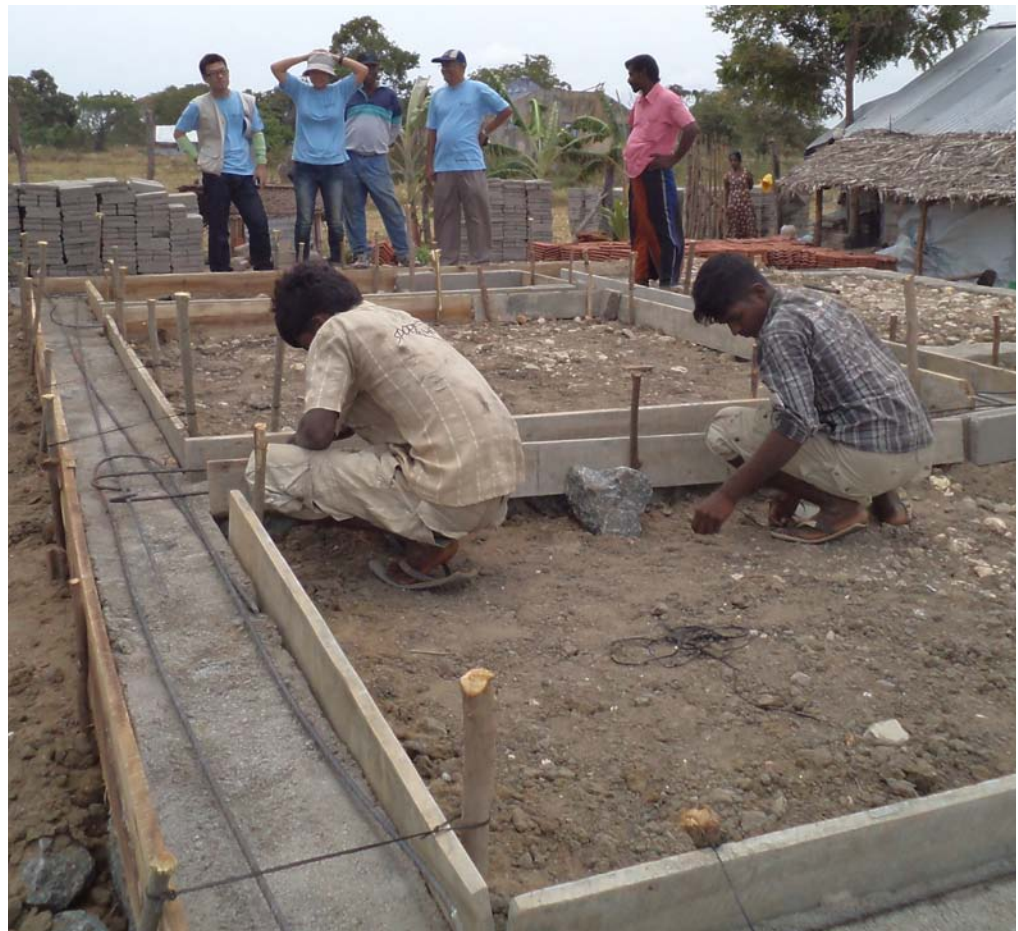
Right: Volunteers and beneficiaries lay a foundation for a new core house.
