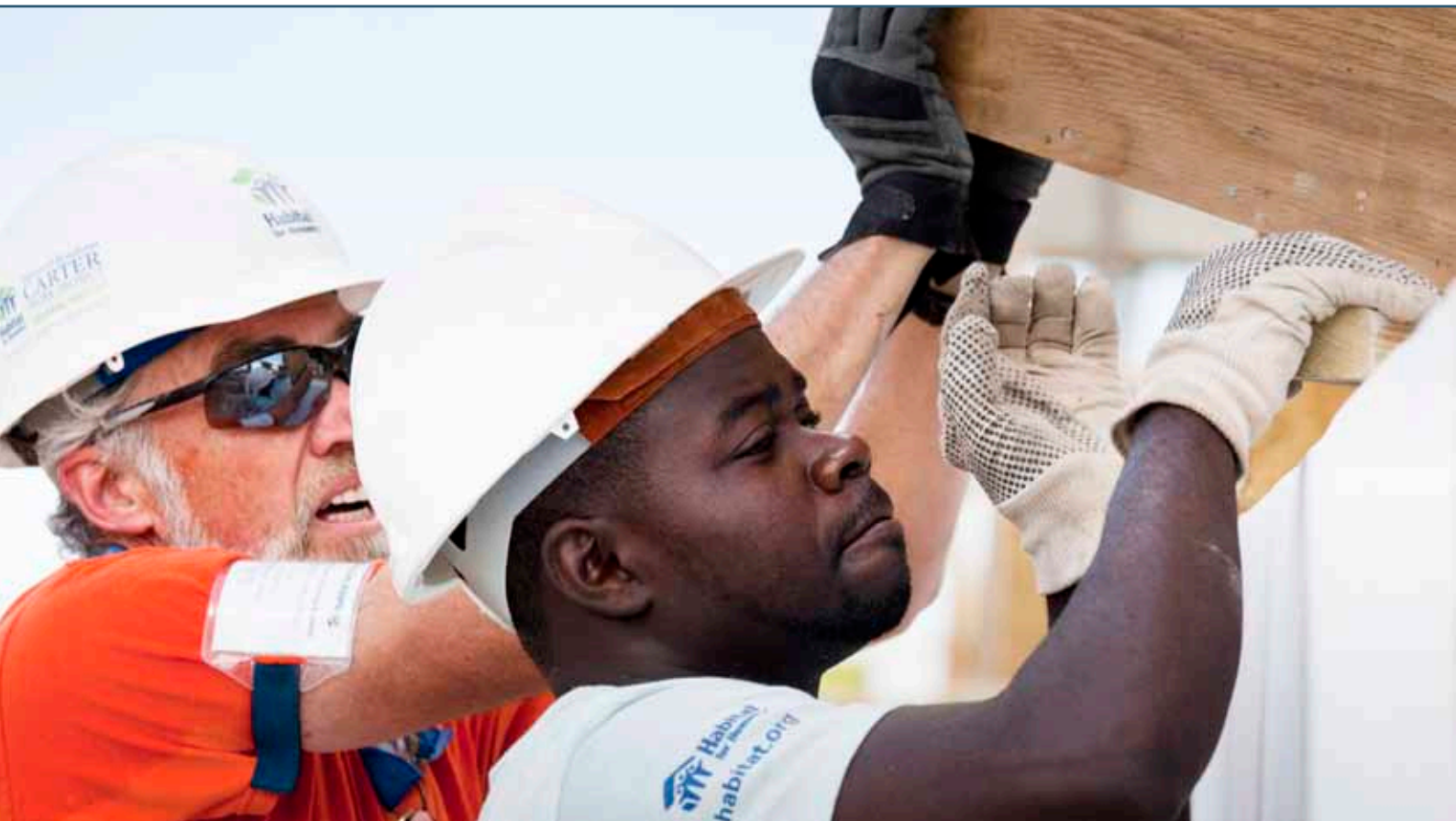
Wiline Dorcelian works alongside volunteers to help construct his Habitat for Humanity home.
